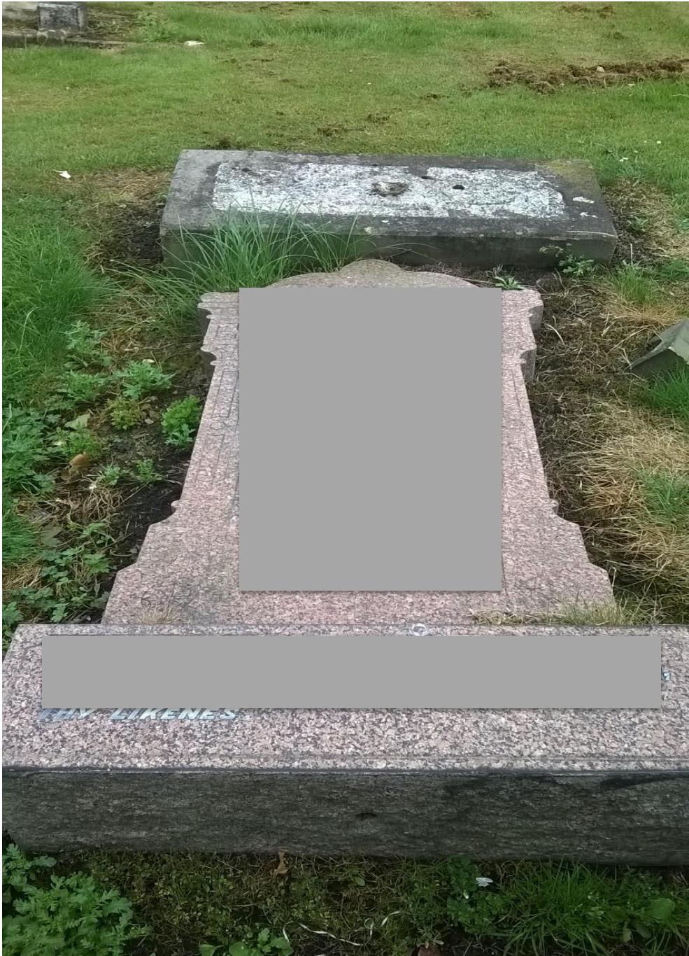
Example of an unsafe memorial, with no dowels, laid flat on the existing grave space.
