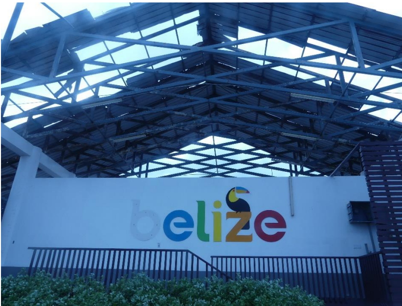
Hurricane damage, Belize City
